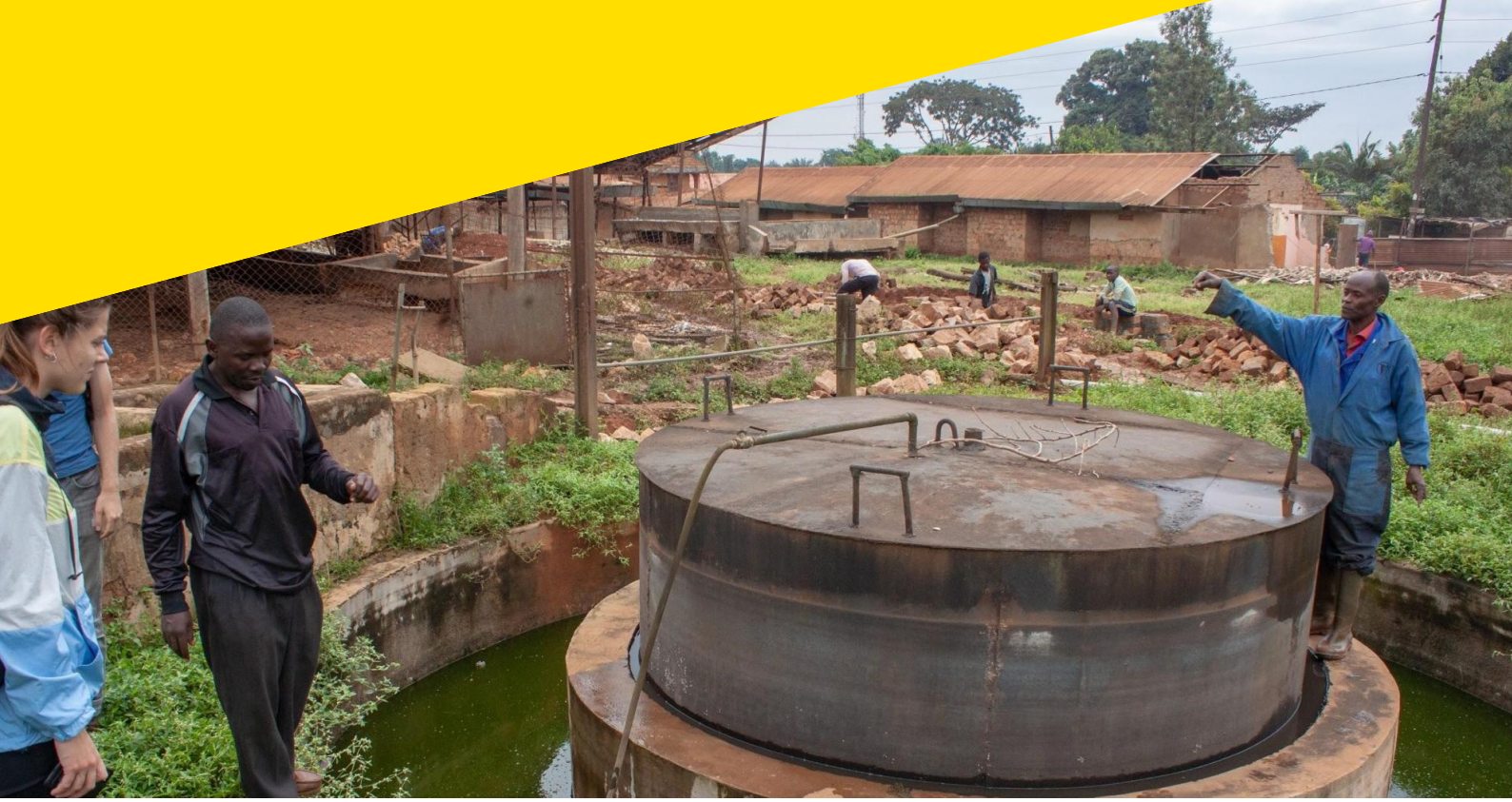
The HS Green Energy Engineering project: carrying out a feasible business model based on social research and completing the optimised design of a fixed dome biogas digester
